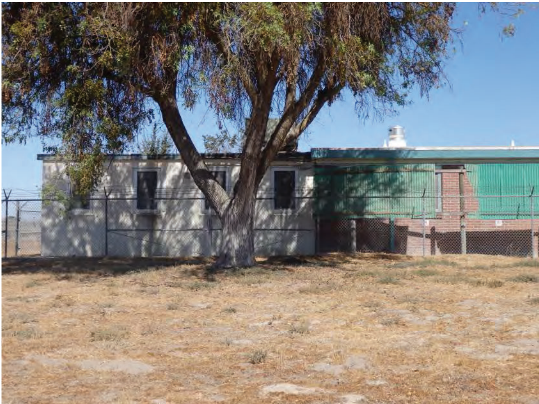
An addition measuring approximately 30 feet by 30 feet was constructed at the west end after 1994.
