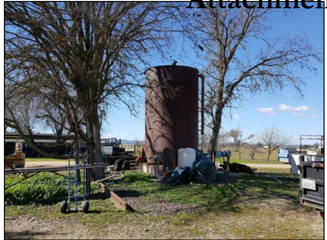
Photo 14: Water storage tank.
