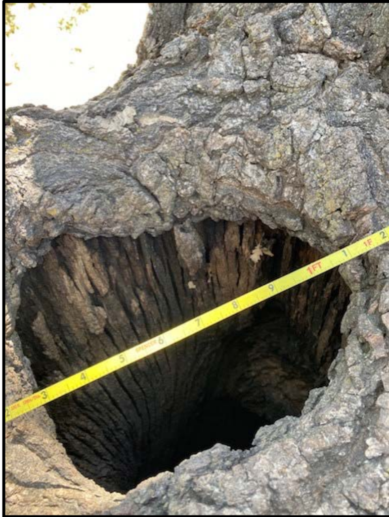
Photo 11 - Tree 2 view of decay cavity formed by failed scaffold. Opening measures 13"
