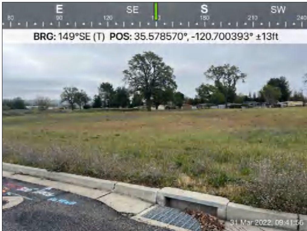
Photo 6. View of storm drain and culvert to direct flow from Nutwood Circle into shallow drainage basin located off-site (north) of the Project Site.
