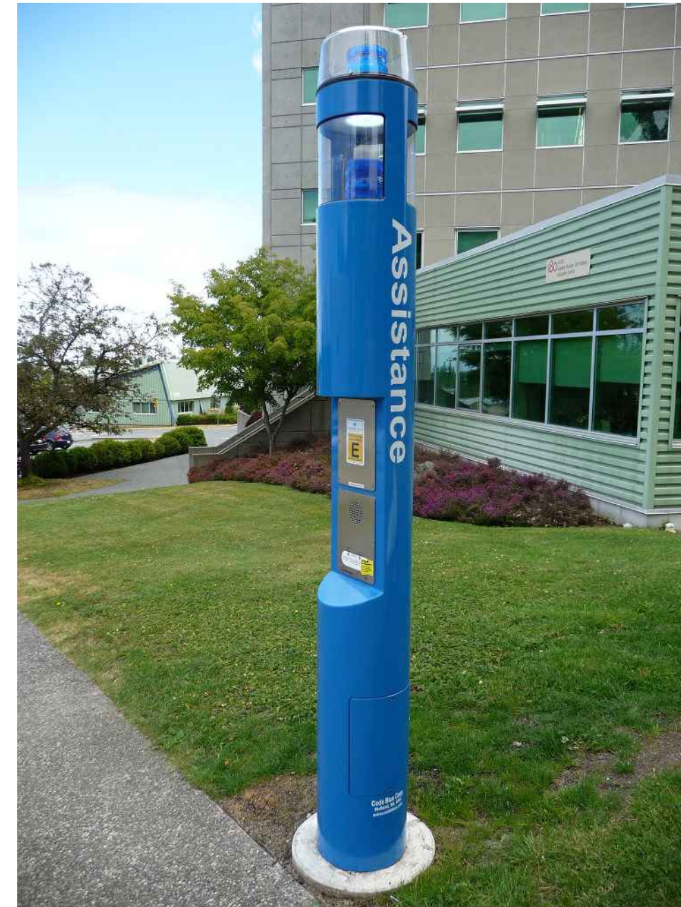
EMERGENCY CALL STATION
